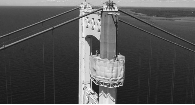
The movable scaffold system designed by Ruby+Associates of Bingham Farms, fabricated by Moran Iron Works of Onaway, and used by Seaway Painting of Livonia, not only allowed that job to be done efficiently on both towers of the bridge, but also earned a structural engineering award in competition with many other impressive projects. Photo courtesy of MDOT
